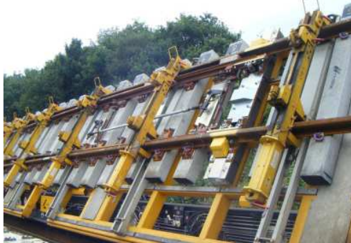
Figure 13 Point operating equipment preinstalled on panel. [Steven Pearson]
